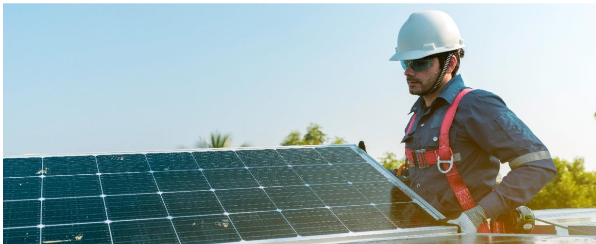
Figure 9: Shutterstock image of solar panel.
