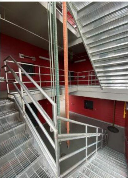
Training tower for repelling, can spray water all over, grate flooring (capture for landscaping?), hang hoses to dry, confined space training, Denver Prop technique
