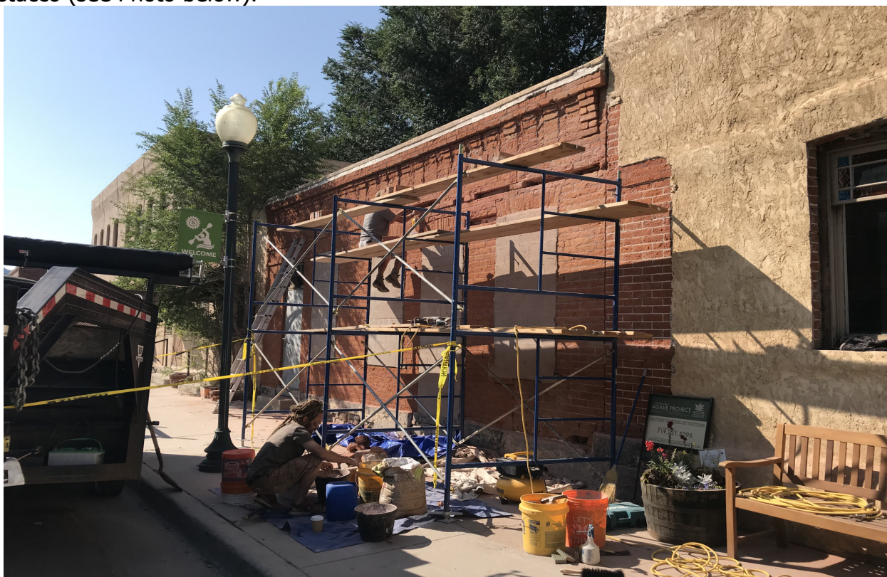
Photo 3: Early in reparation stage. Note damage to original upper band and cornice dentil detail.
