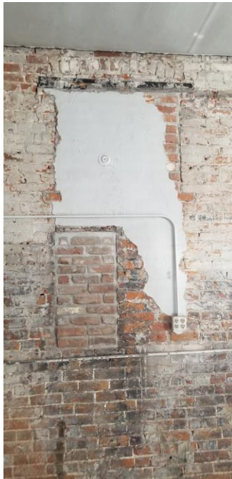
Image #7 (below), In-filled window at Alley, view from interior. Expose and replace.
