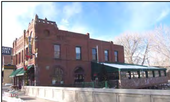
228 N. F St, Bon Ton Hotel, Manhattan Hotel – The addition on the rear and side can be differentiated as new rather than historic.
