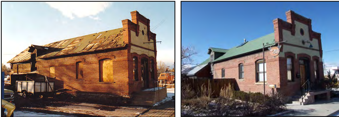
211 W. First Street, Salida Bottling Company – Before and after rehabilitation. Now used as a private residence.
