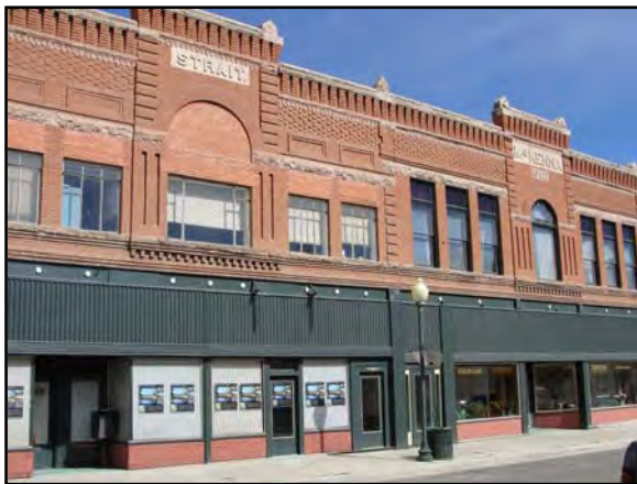
230 F St, McKenna Building – The left side of the building has undergone an inappropriate window replacement.
